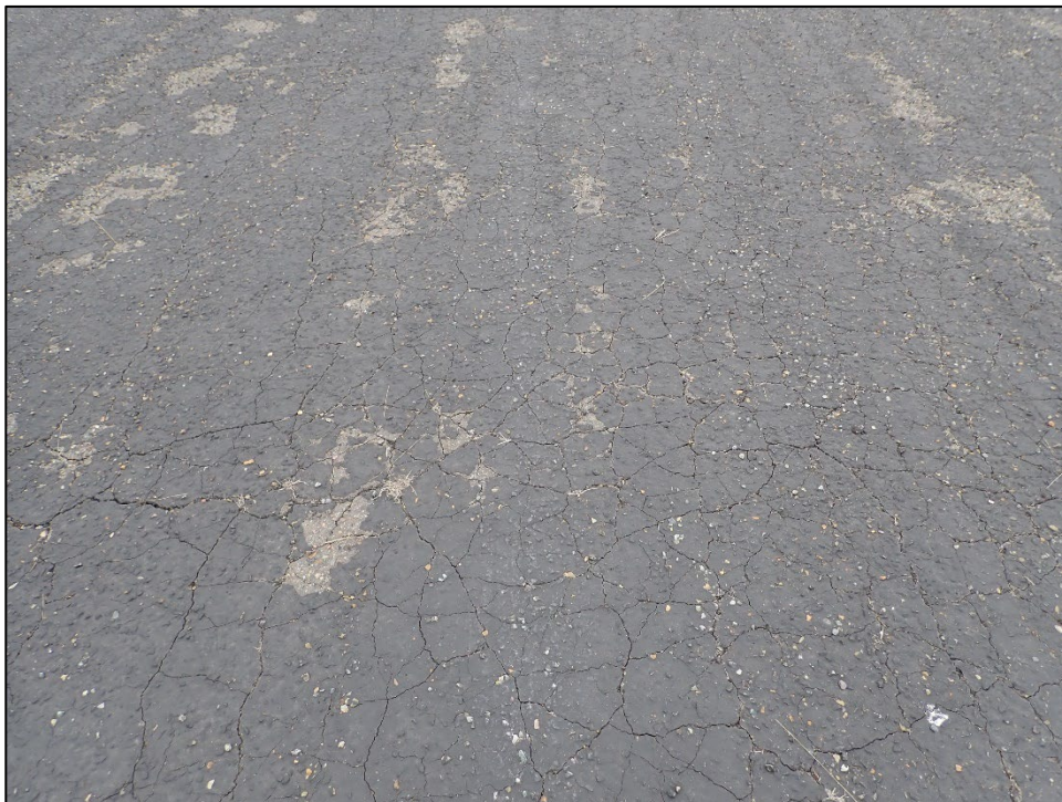
TW-01-02: Alligator Cracking
