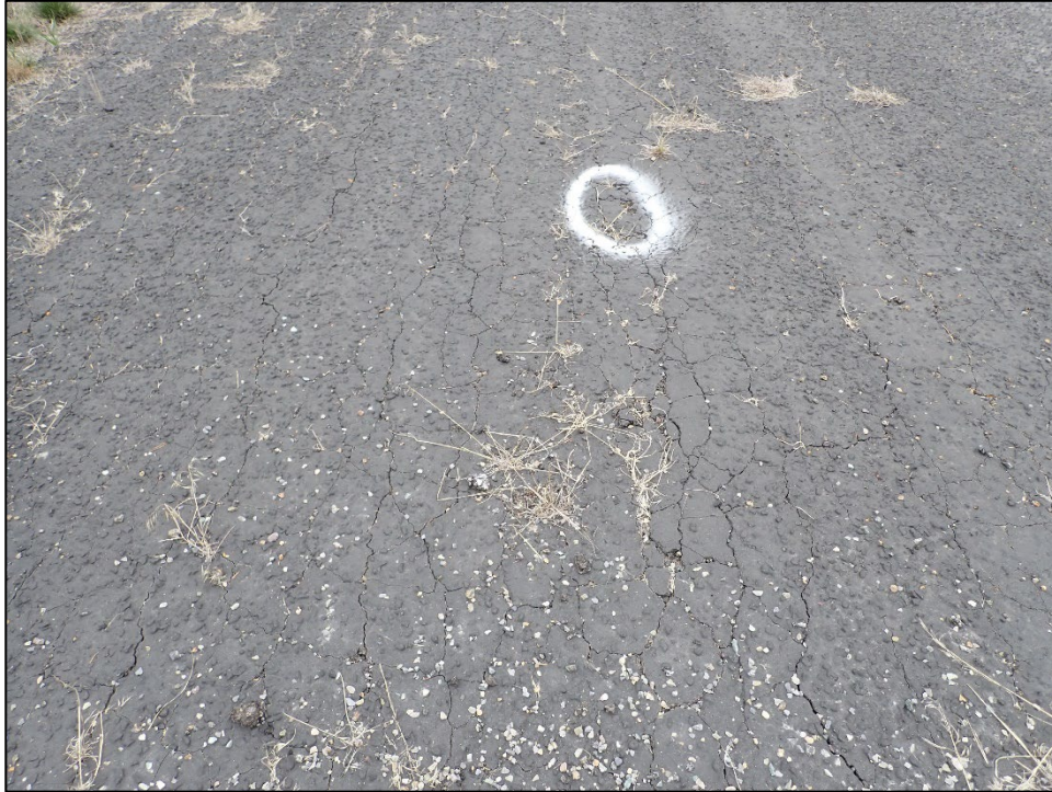
RW14-01-02: Alligator Cracking
