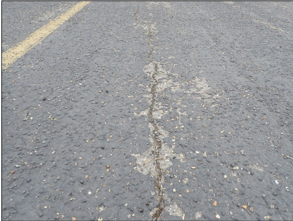
TW-01-01: L&T Cracking
